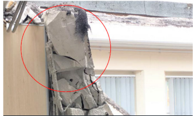
Figure 3. A roof slab collapse constructed with RAAC
