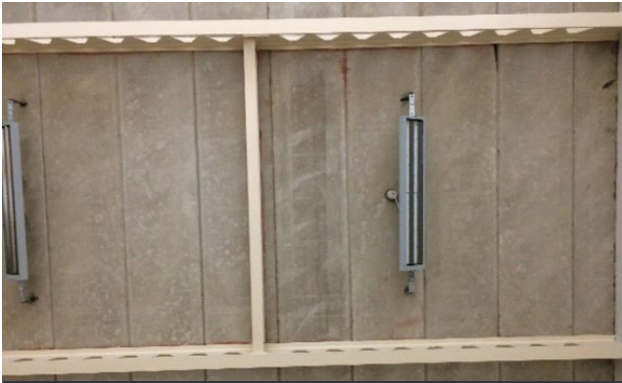
Figure 2. Exposed RAAC panels.
